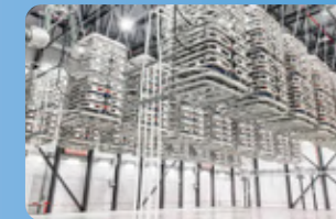
Example: HVDC conversion plant for the mass adoption of renewable energy
